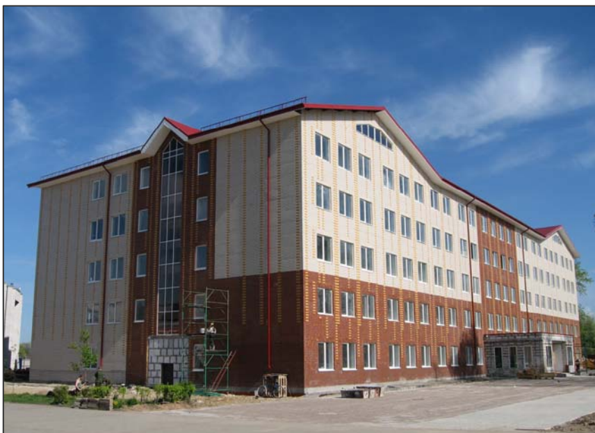
Part of the replacement construction work for the Russian military, within the Moika/Glinki agreement
